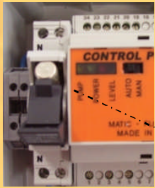
BIPOLAR 32 A ON/OFF switch complete with FUSE
